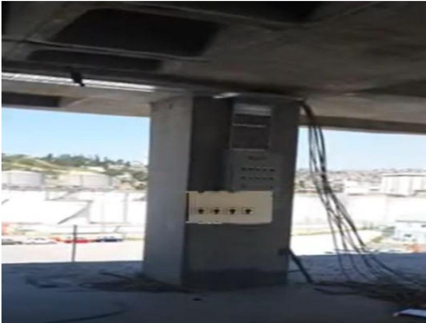
Figure 7. Inappropriate electrical wiring in the parking area
