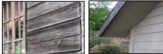
Figure 10-11. Home on left is vulnerable to wildfire because of its aging, shrinking wood siding and single pane windows. Home on right was retrofitted with fire-resistant siding, boxed eaves, metal-clad fascia and double paned windows (Sonoma, 2004).
